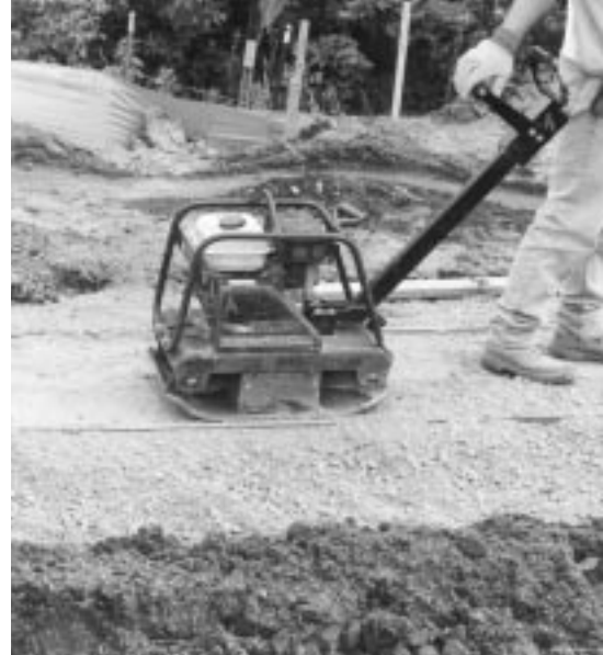
Compacted granular leveling pads provide stiff but flexible bases for Mosaic units.
